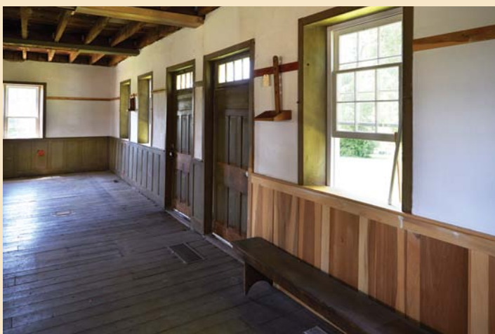
Wainscoting. Volunteers Joe Grittani and Dave Coleman made and installed replication poplar wainscoting to replace the many missing sections on the first floor of the meeting house. At the back of the picture, you can see original panels; the unpainted sections are new. Notice, too, the open ceiling; all the plaster had to come down to rip out old wiring and to install joist hangers that support 100 pounds per square foot.
