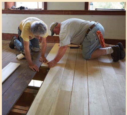
Flooring. By the time this is printed, Joe and Dave will be finished installing custom-milled poplar planks that match the original flooring. The plan is to wash the old floor then use the dirty water to "stain" the new floor so that they more closely match.
